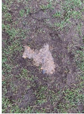
Fig.5: Exposed concrete rubble (R Challoner)
